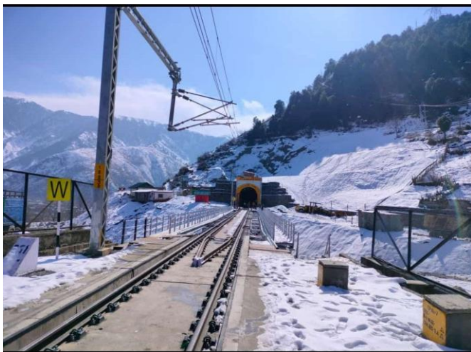
Figure 7: T78-P2 after commissioning
